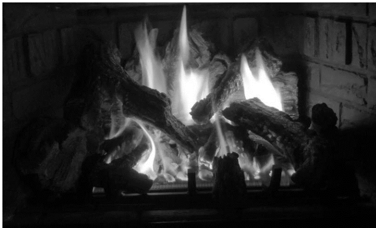
Figure 6-2 Burner Flame Heights: This image provides a visual reference for the burner flames burning at maximum height after the burners have been operating for 30 minutes or longer. A normal rear flame will be 1 to 2 inches above the rear log top edge. This, however, is dependent on the gas type, air shutter opening setting and vent system configuration. Actual flame heights can be slightly higher or lower when compared to this reference image.
